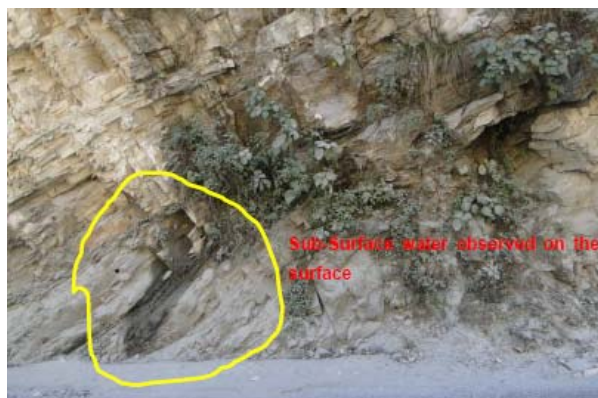
Fig. 9. Water seeping through jointed rock-mass
