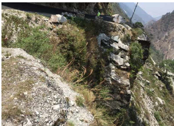
Fig. 8. Foliated rock & blocks of rock below road level
